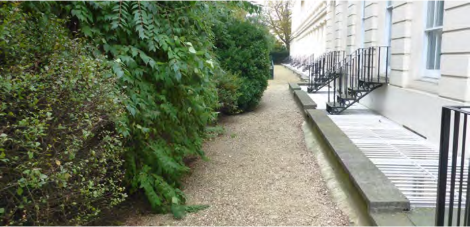
Left: An existing gravel path runs the length of York Terrace East. The path appears to be suffering subsidence, evidenced by the exposed concrete.
