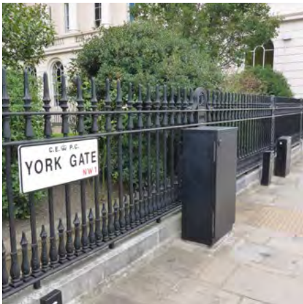
Left (York Terrace East): Piecemeal repairs to damaged railings are present along the length of the terrace.
