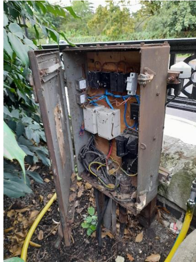
Figure 3-3 - Existing supply point at Cambridge gate.
