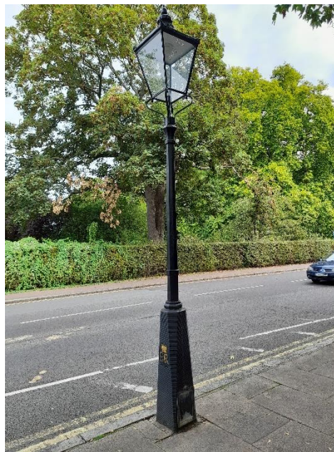
Figure 4-4 - Existing CEPC Lighting Column
