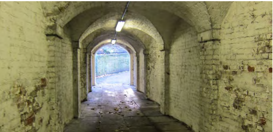
Right: View within the tunnel showing damaged lime wash, poor 20th century lighting and crack paving
