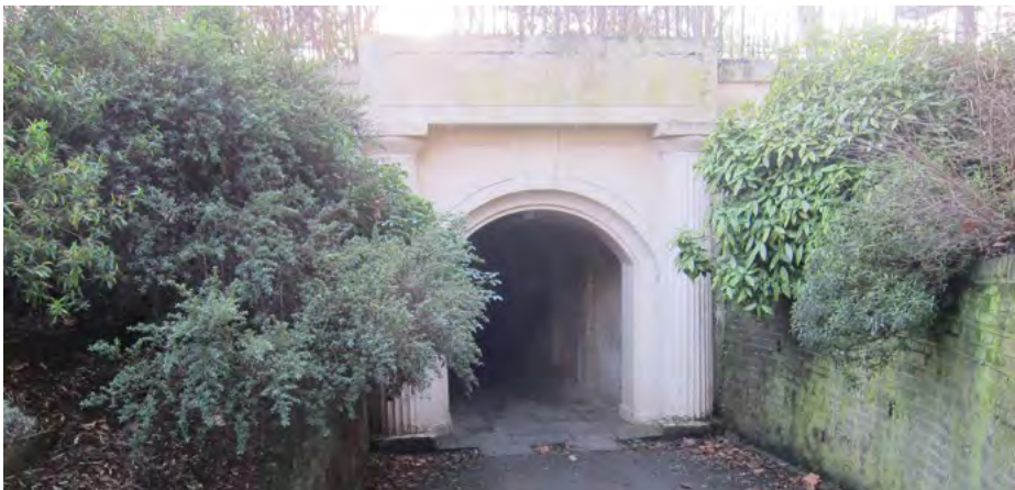
Right: The north headwall requiring concrete strengthening
