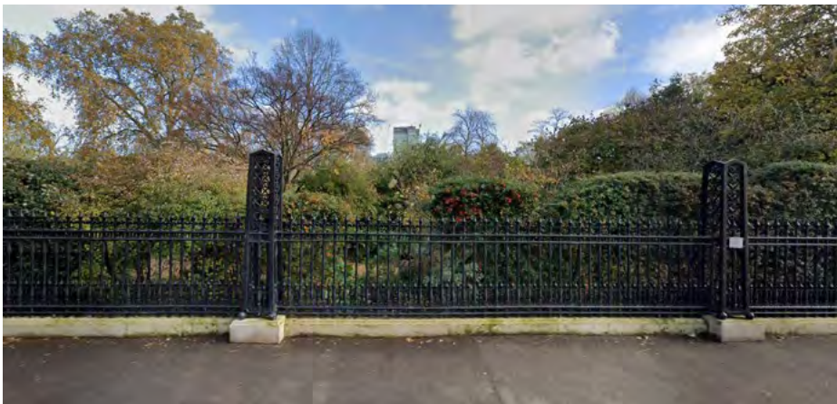
Right: Existing railings along Park Square West. The perimeter railings across Park Square and Park Crescent use the same Nash design featuring cast iron Grecian spear head railings between openwork obelisk standards. Only the sections adjacent to the main roads are distinct, as they feature lanterns placed atop the obelisks.
