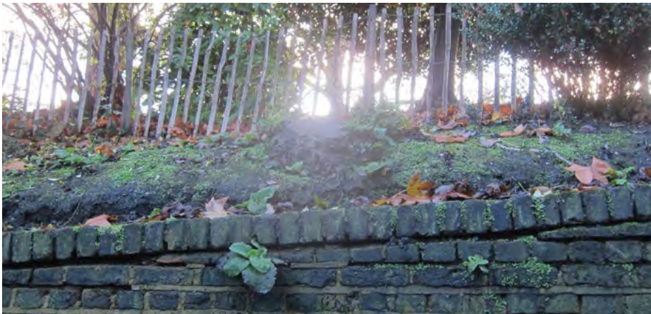
Right: Deteriorating historic brick wall and soils eroding over the top of wall along the ramp leading to Nursemaid’s Tunnel in Park Crescent.
