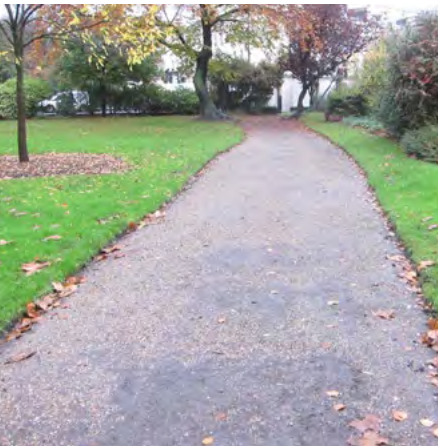
Far Right: Muddy paths likely caused by compaction of sub-base and subsequent lack of drainage
