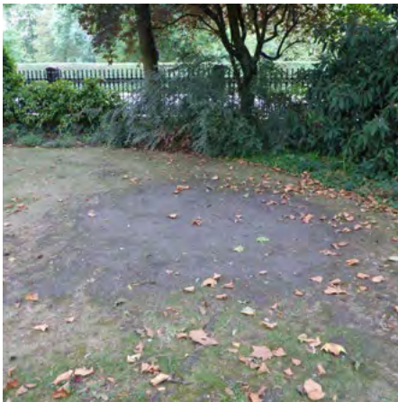
Right: Bald and muddy patches in lawns caused by poor drainage.
