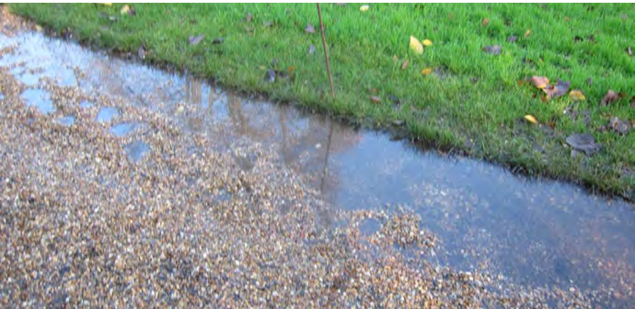
Left: Drainage issues affect the paths, likely caused by malfunctioning drainage system and compaction of path sub-base.
