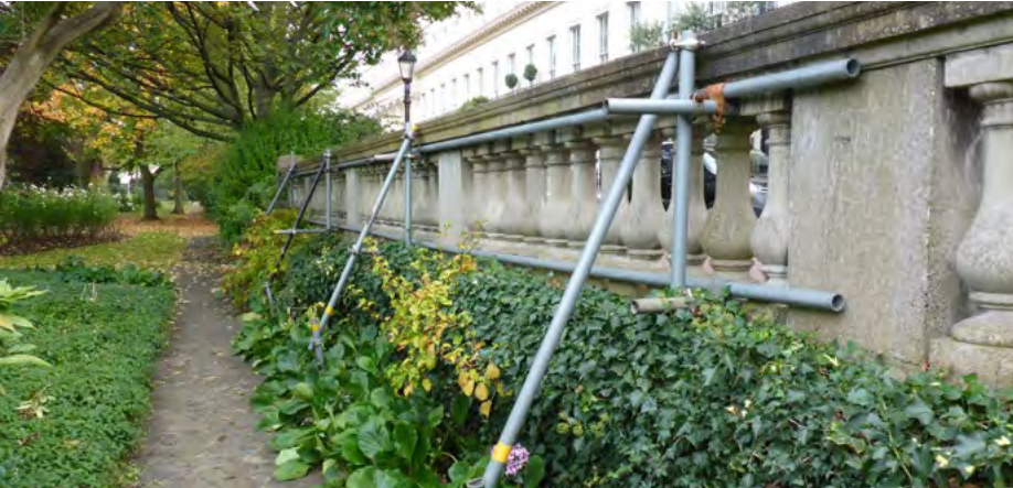
The existing concrete balustrade at Chester Terrace is in a poor state of repair and requires urgent refurbishment to ensure it is structurally sound.
